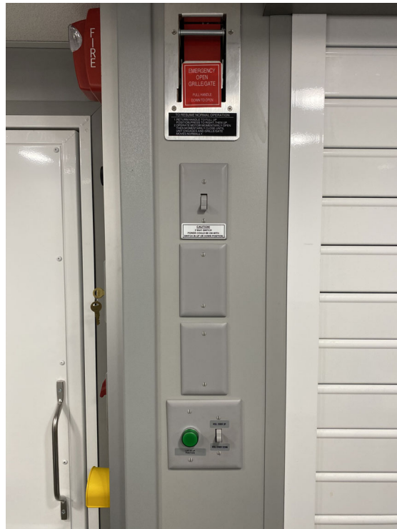
Figure 33: Roll Door Emergency Release
