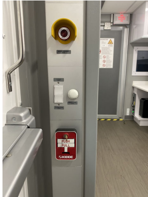
Scan Room Lighting
