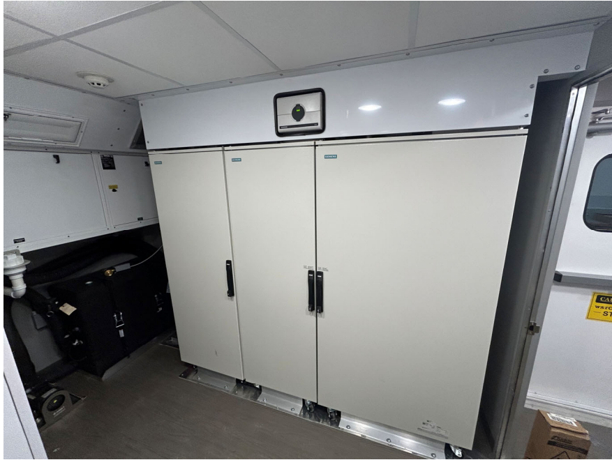
Figure 6: Cryogen Compressor Cabinet
