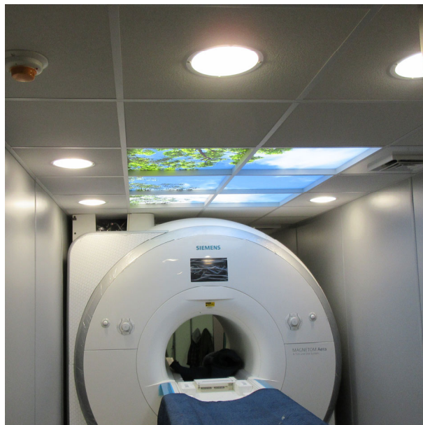
Figure 60: Scan Room Lighting
