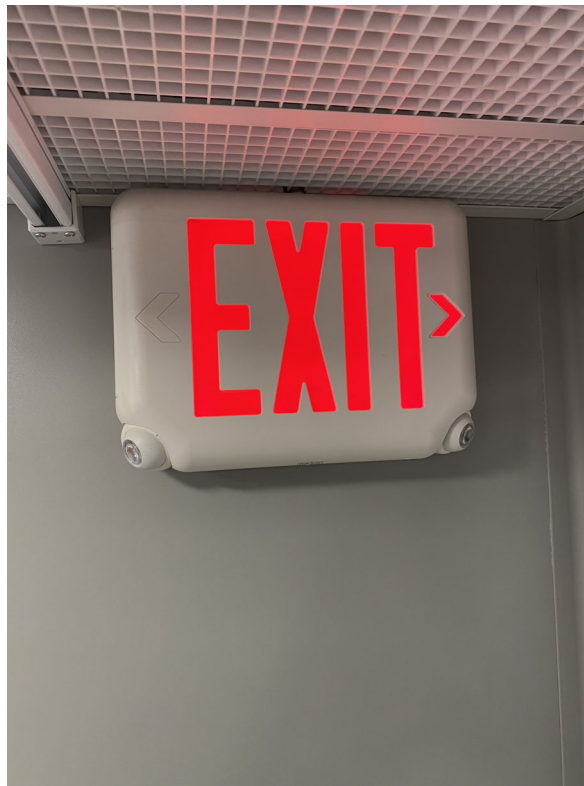
Figure 54: Emergency Dual Beam Lighting
