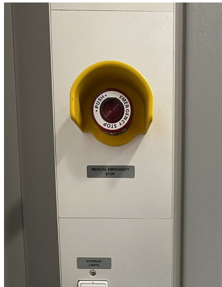
Emergency Off button, Control Room, next to Entry Door
