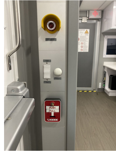
Emergency Off Button, Magnet Room
