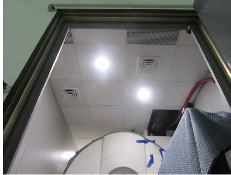
Figure 61: Scan Room / Magnet Room Lighting and Switches
