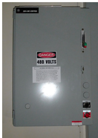
Figure 37: A1 Electrical Panel
