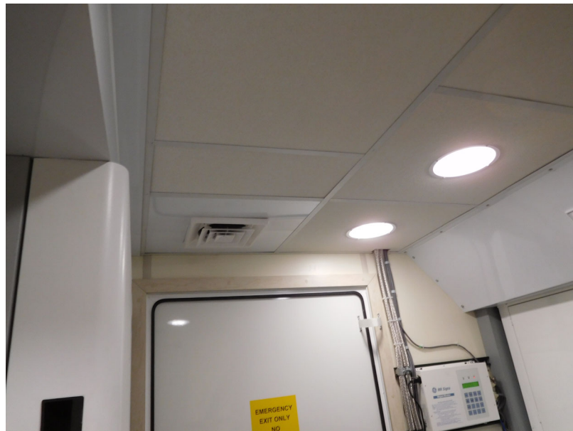
Figure 58: Equipment Room Lighting
