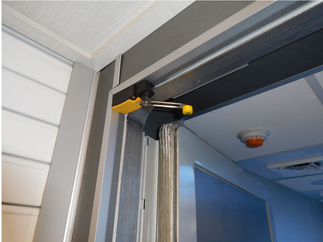
Figure 64: RF Shielding Close up of RF door trim
