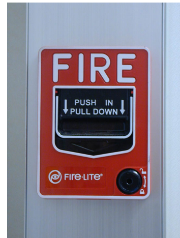
Figure 28: Fire Alarm Pull Station
