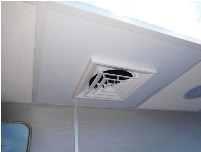
Figure 47: HVAC Components HVAC Vents Discharge
