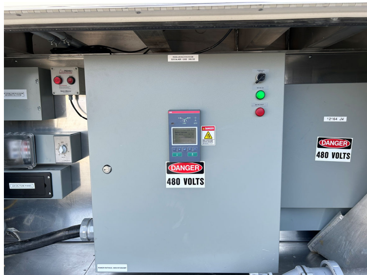
Figure 11: Power Supply Control Panel
