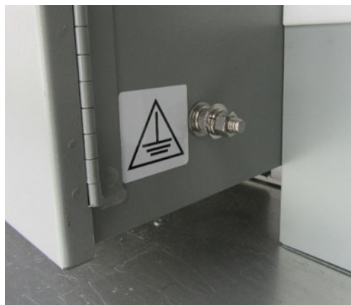
Figure 40: Power Supply Control Panel Ground Connection
