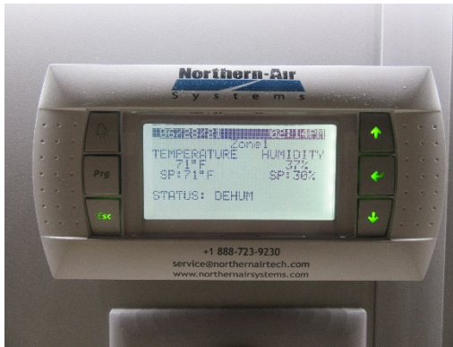
Figure 16: Mobile Unit Controls HVAC Monitor & Alarm
