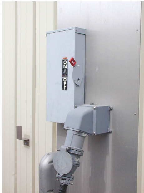
Figure 38: Shore Power Connection
