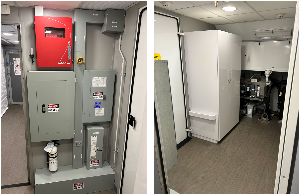
Figure 8: Equipment Room Overall
