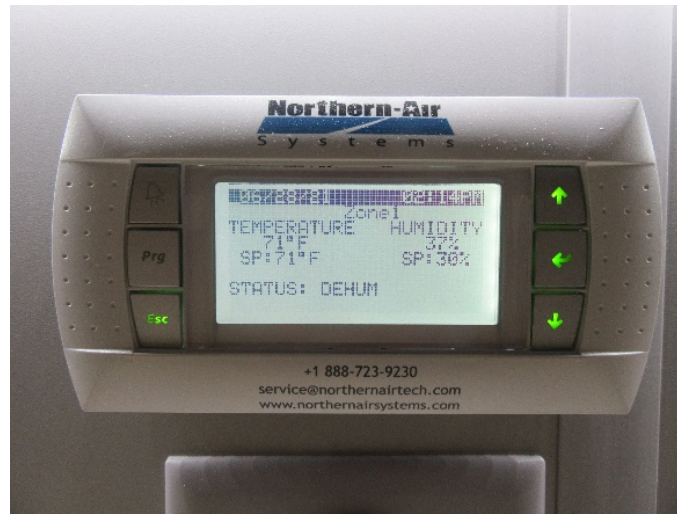
Figure 44: HVAC Monitor and Alarm Panel
