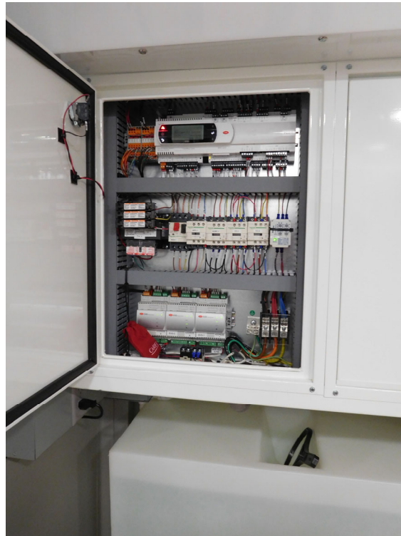
Figure 43: A/C / Chiller Control Panel
