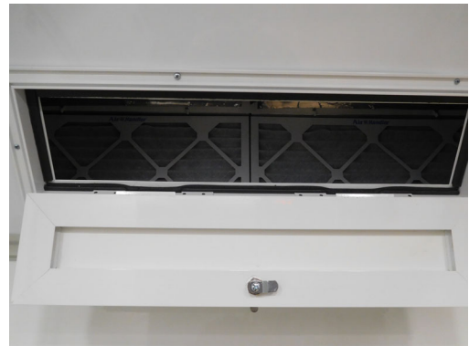
HVAC Filter Access
