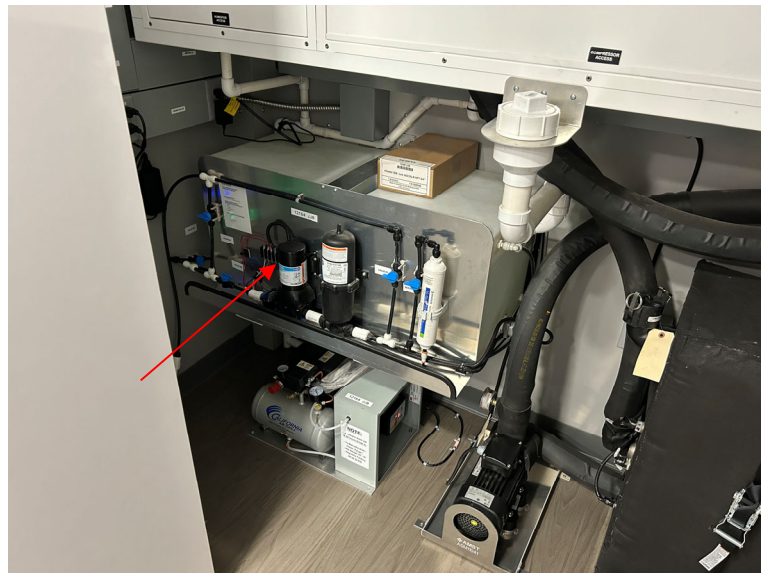
Figure 45: Humidifier Water Tank
