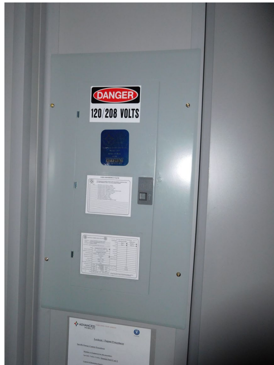
Figure 24: 120/208V AC Electrical Panels
