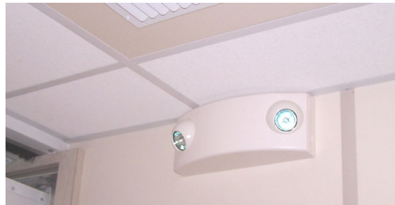
Gantry Room Emergency Light
