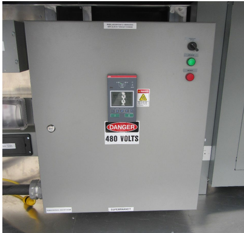
Figure 22: Automatic Transfer Switch and Phase Power Monitor
