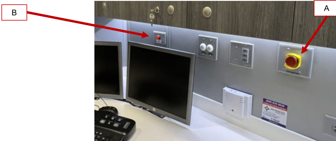
Figure 4: Control Room Overall
