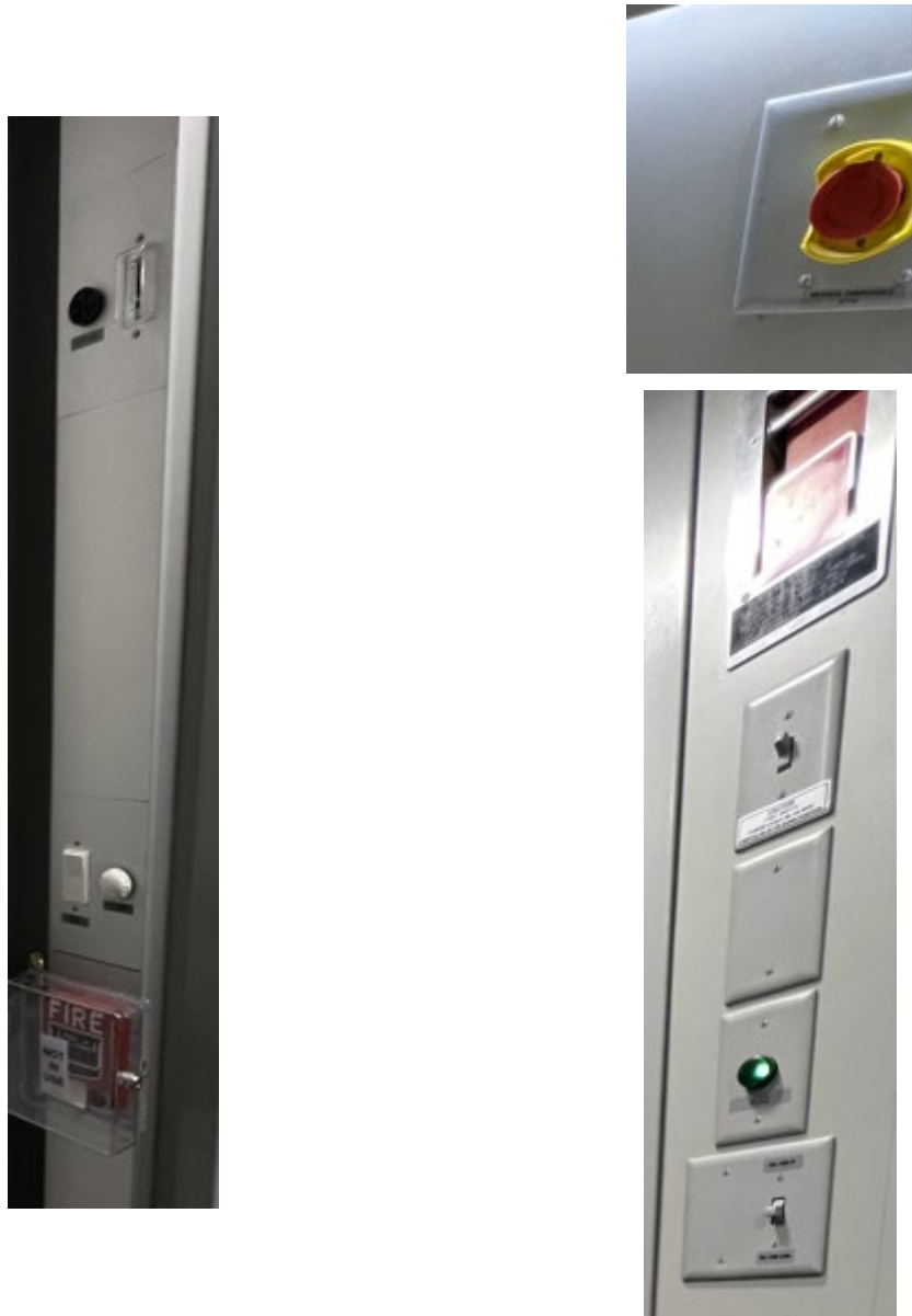
Figure 11 Mobile Unit Controls
