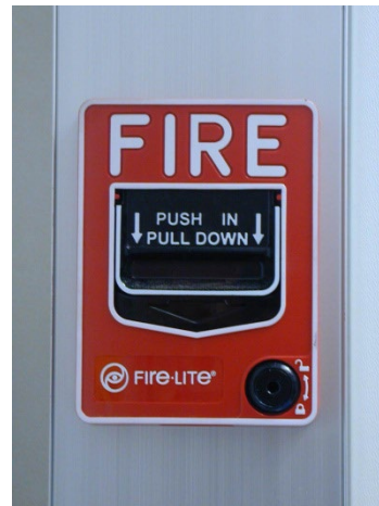
Figure 20: Fire Alarm Pull Station
