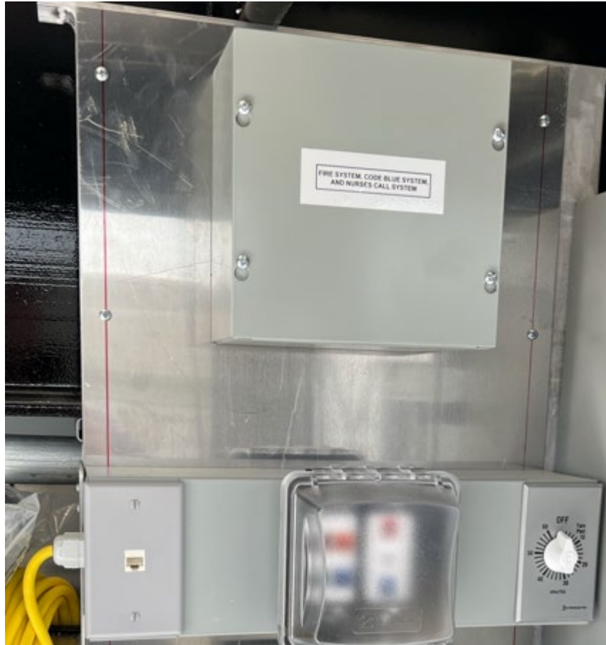
Figure 12: Phone & Data Line Connections
