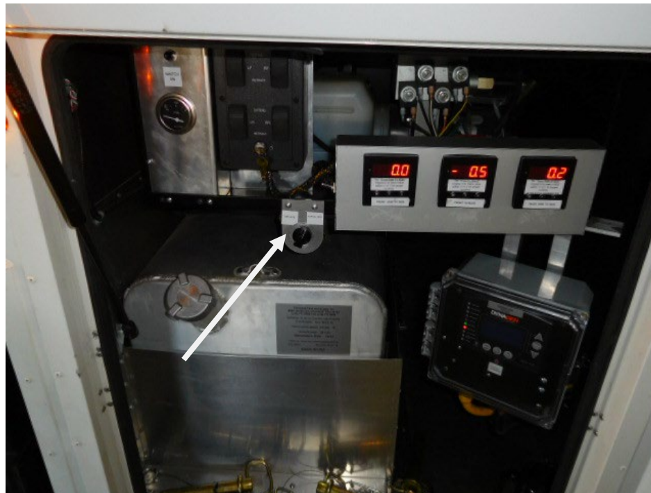
Figure 33: Air Bag Controls
