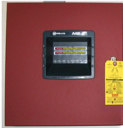
Figure 19: Fire Alarm Control Panel
