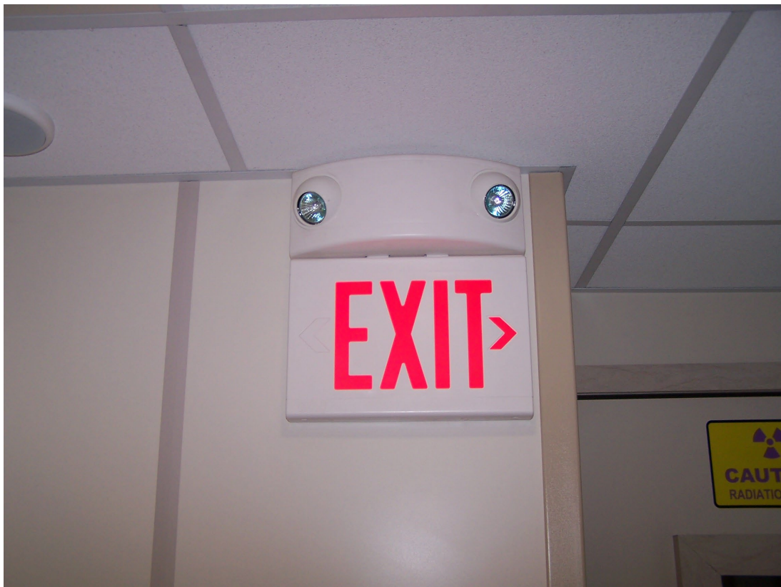
Figure 16: Control Room Emergency Lighting
