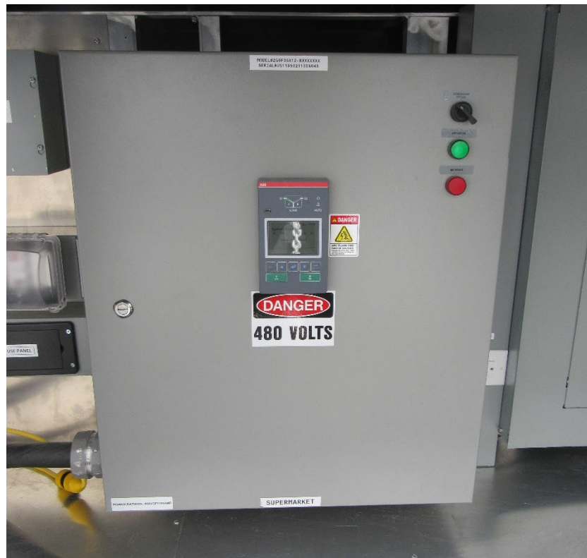
Figure 25: 480V AC ATS and Phase Power Monitor
