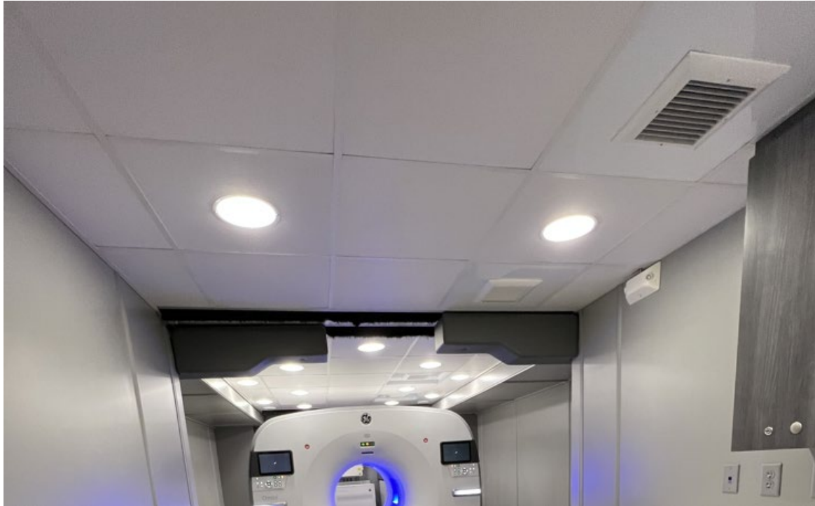
Figure 38: Gantry Room Overall Lighting
