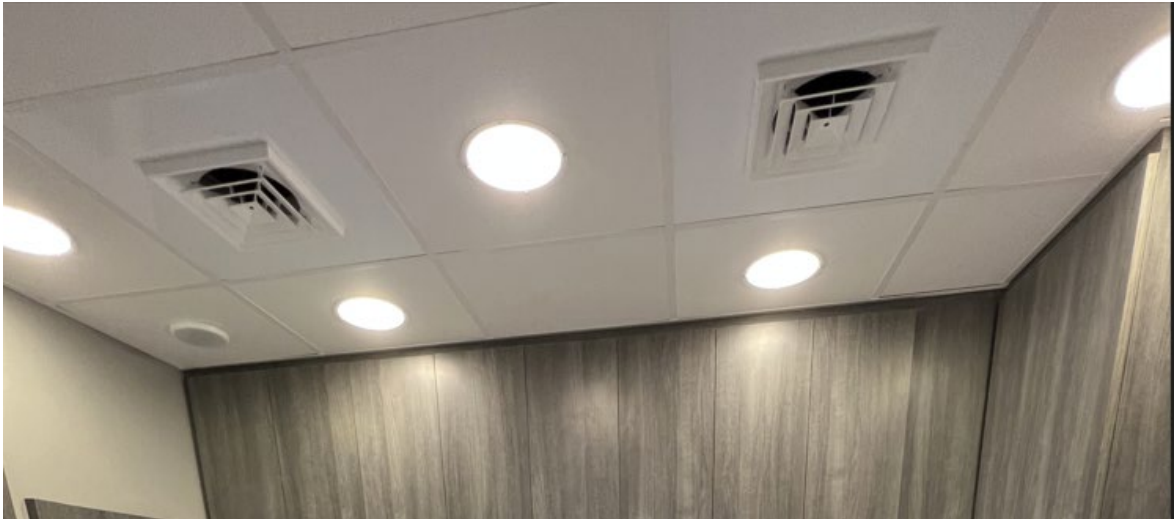
Figure 37: Control Room Overall Lighting
