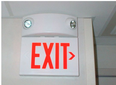
Control Room Emergency Light
