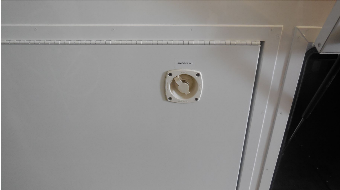
Figure 23: Humidifier Tank Fill
